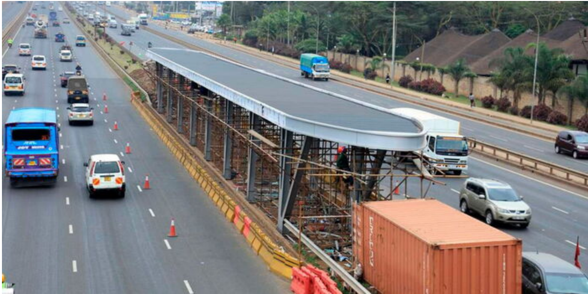
Figure 5: A Bus Rapid Transport (BRT) station under construction along Thika Road at Safari Park footbridge. Source: Kenha.
