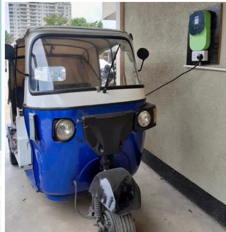
Figure 16: Charging station for e-three-wheelers at DIT
